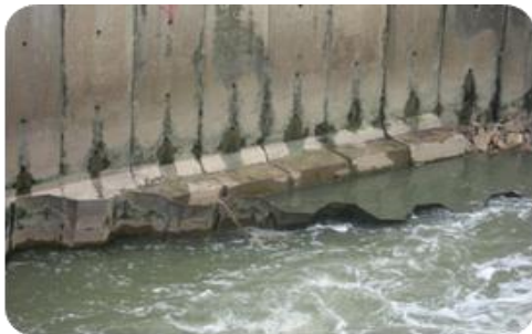
Rajah 2.3(f): Runtuhan Sheet Pile cut-off
