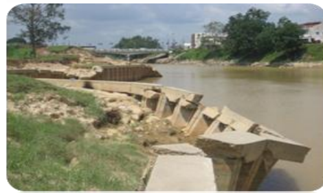
Rajah 2.3(e): Runtuhan Tembok Sheet Pile
